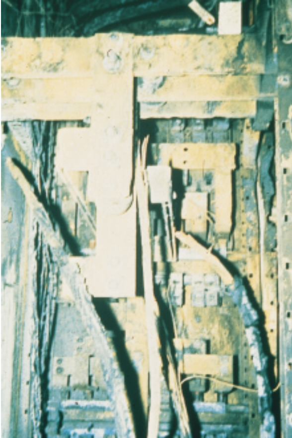
This burnt out switchboard represents the staggering monetary losses in equipment and facility downtime that can result from inadequate or deteriorated protective devices. It emphasizes the need for reliable protective devices that properly function without progressive deterioration over time.
